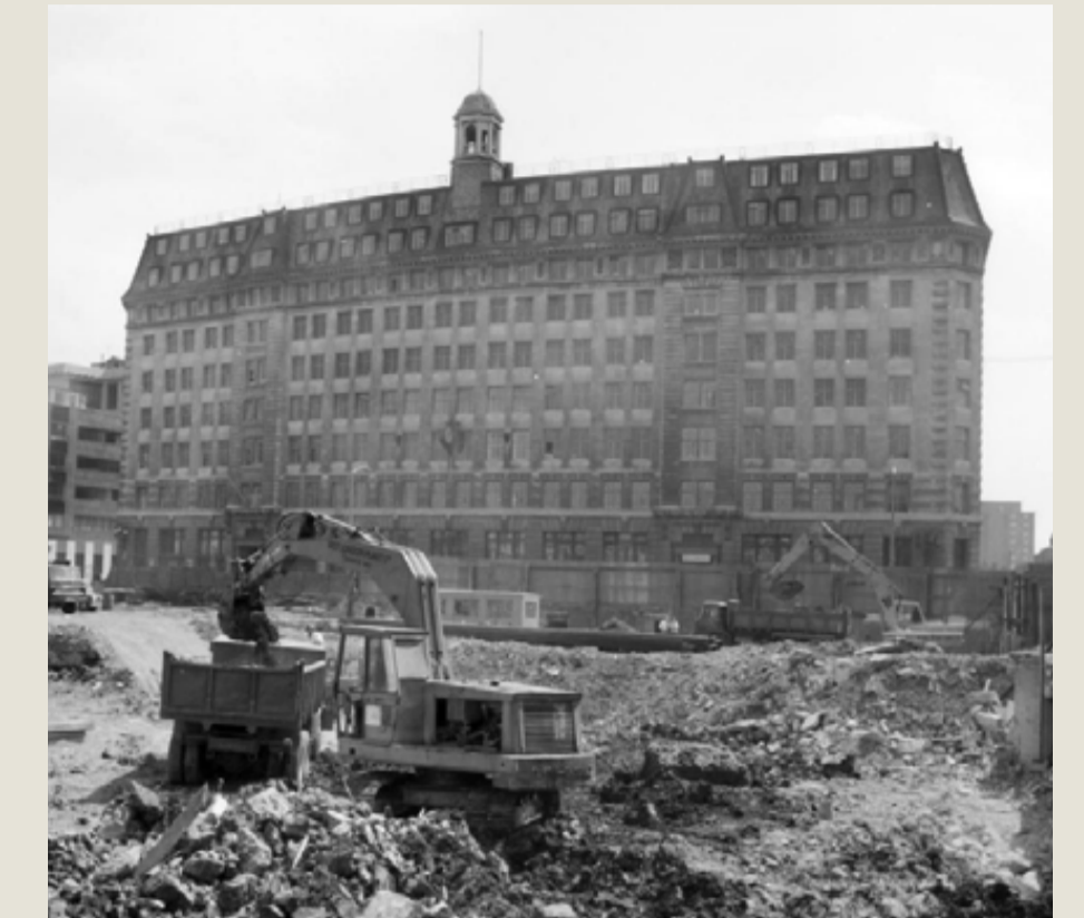
View of Dorset House from Stamford Street, Southwark, at the junction with Hatfields. At the time this photo was taken, Dorset House, an eight-storey office building, was occupied by IPC Business Press Office.
