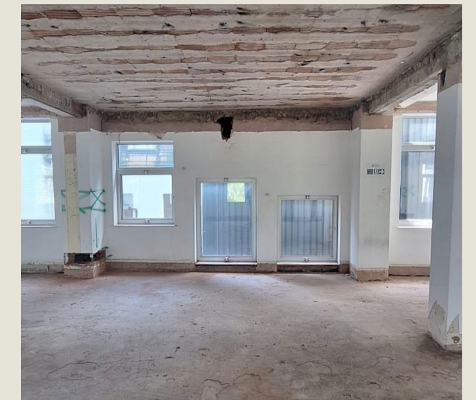
Degraded structural elements
